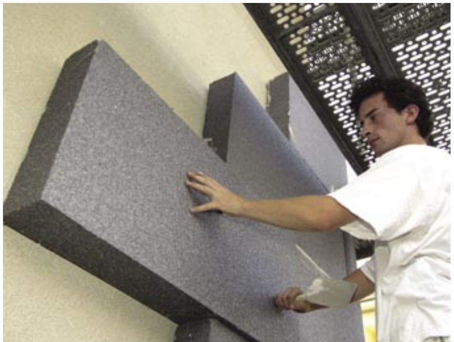
Neopor is bonded on the facade. The craftsman fixes the insulating board by pressing on firmly by hand. The insulating material is then secured with screw anchors.
